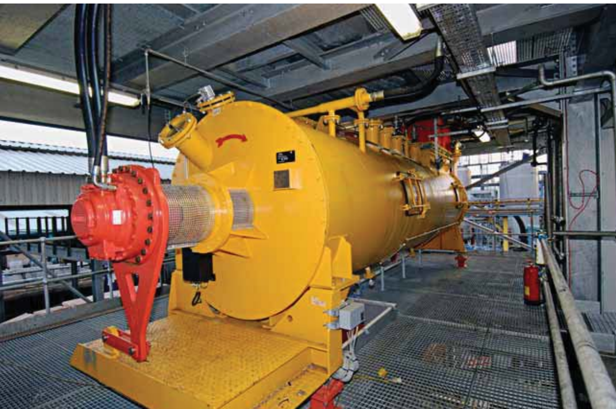
2 Mixing equipment for continuously setting of chemical and physical properties
